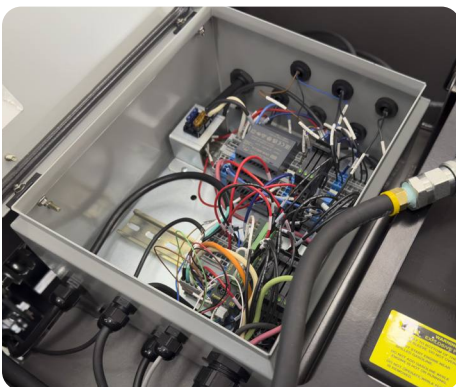
Larger Accessible Electrical Box
