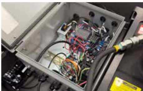
LARGER MORE ACCESSIBLE ELECTRICAL BOX
